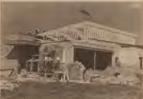
Student builders of the Professional Development Center reached the building's high point in September, and topped it with the traditional tree.
